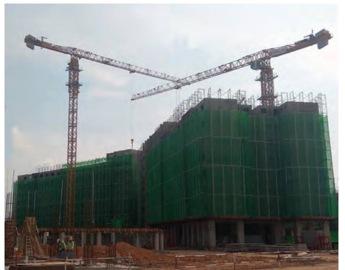
Megah Sewa has added three Potain MCT 385 topless tower cranes to its fleet for the first time. The units have been deployed on residential projects in Kuala Lumpur and Sepang, Malaysia.
