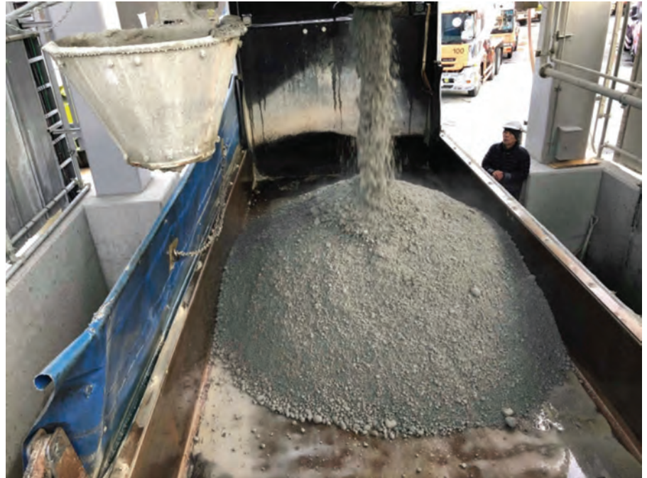
ABOVE: The production phase of roller compacted concrete (RCC) that would be used to build a new carpark at the Panorama Park cable car station, located in the town of Izu Nagaoka.
