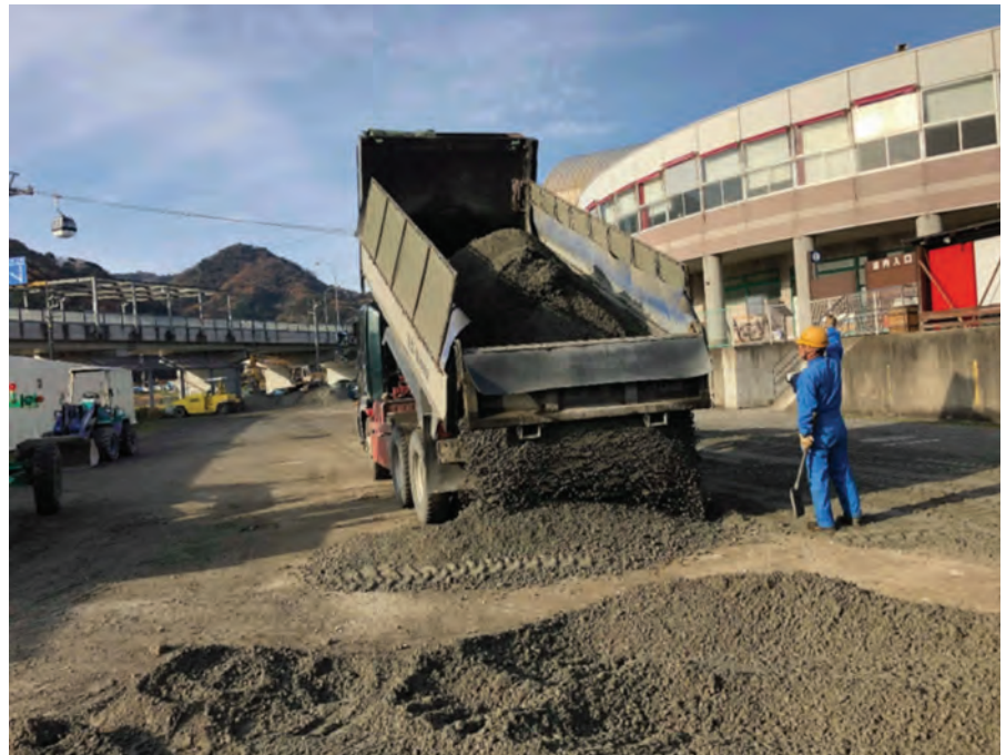
BELOW: Once mixed, the concrete was transported and distributed on site in layers of between 10- and 20-cm-thick, before the compaction phase started.
