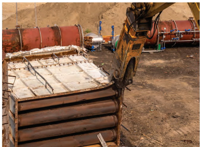
ALL IMAGES: Indeco ISS 10/20 shears being deployed on a renovation project at the gas storage facility in Minerbio outside Bologna, Italy.
