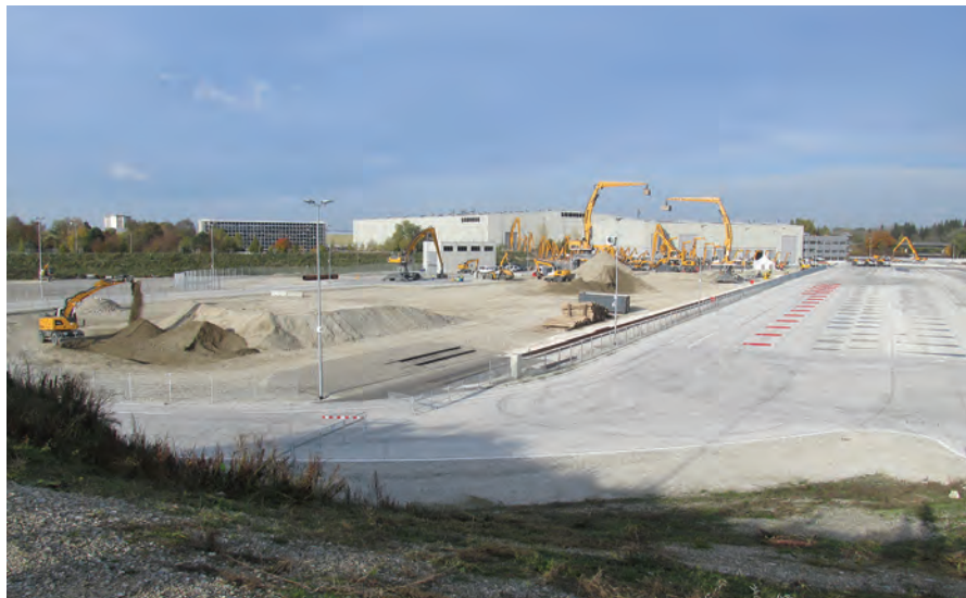
The Kirchdorf development and demonstration centre serves as the development and testing ground for Liebherr earthmoving machines and material handlers.
