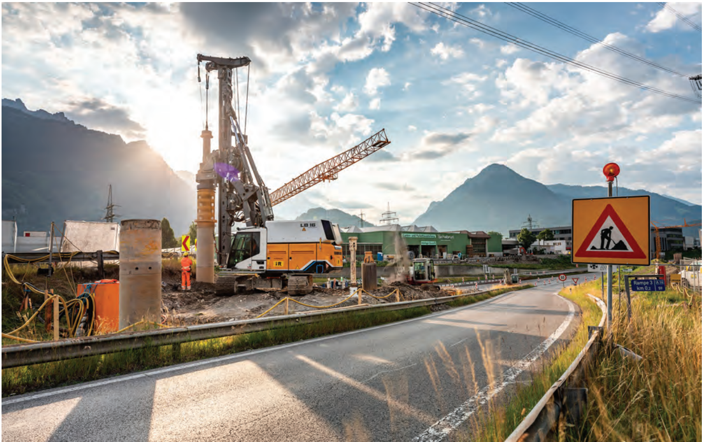
TOP: At the Bludenz-Bürs junction, the LB 16 unplugged was used by local company i+R t to install 148 piles and drill 1,742 m into the ground. The piles varied between 10 m and 14 m in depth, featuring a diameter of 900 mm.
