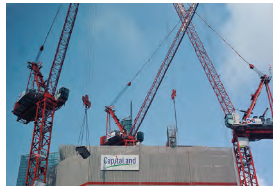
Apart from the Potain MCR 295, the other luffing jib cranes supplied on the project are two units of MR 295 and two units of MCR 225A.
